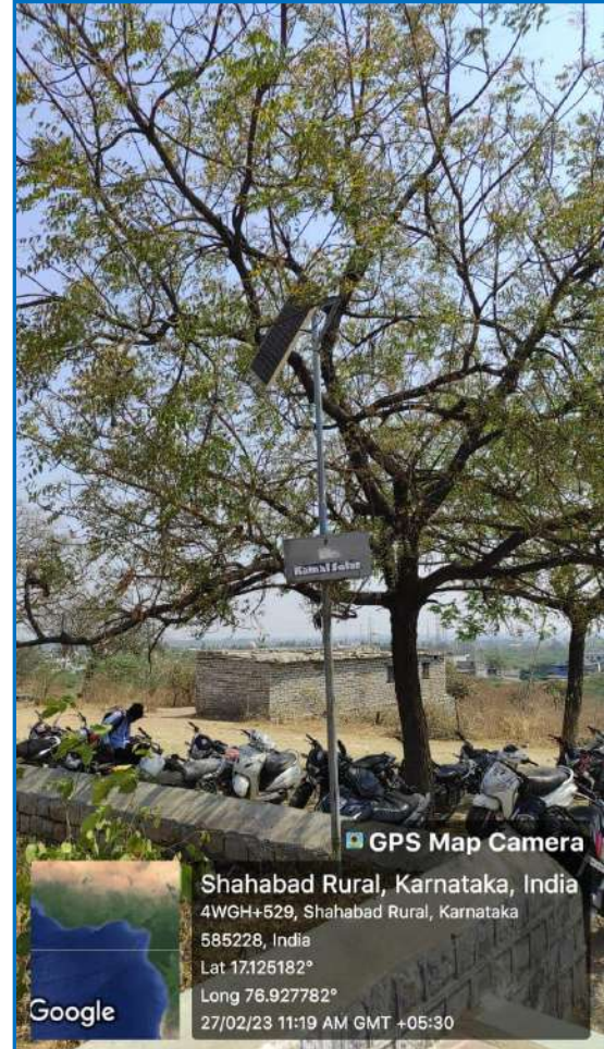
Solar Panel lighting system outside campus
